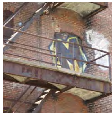
Lovejoy Pl., Boston, MA graffiti obscuring architectural elements
